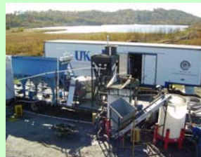
Trailer-mounted pilot test installation.
